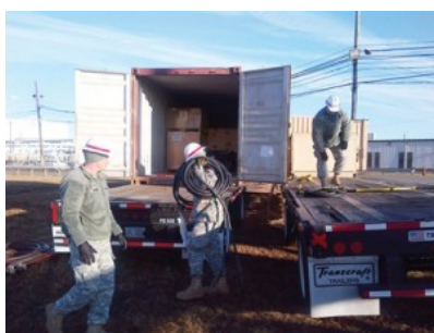
249th Engineer Battalion Soldiers unload power restoration equipment to help return electricity to Northeast region priority facilities.
